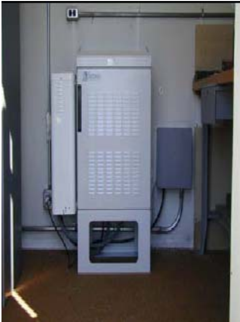
ADS-B Ground Installation the size of an average filing cabinet
